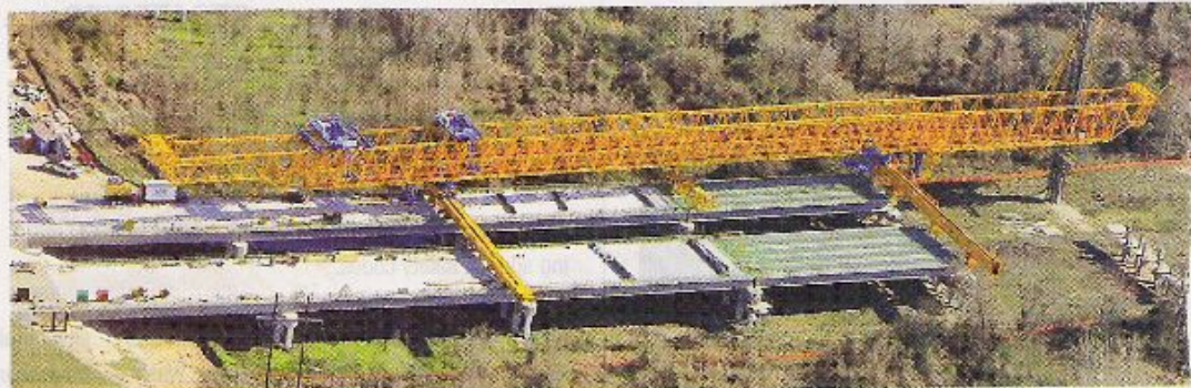
▲ Drive and Launch. Homsy gathered a variety of industry minds to develop his idea of a pile-driving truss.
